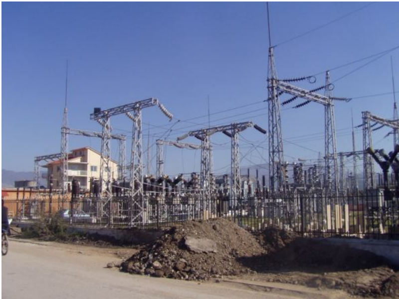
Figure 5: Electric power station of the Industrial Zone
