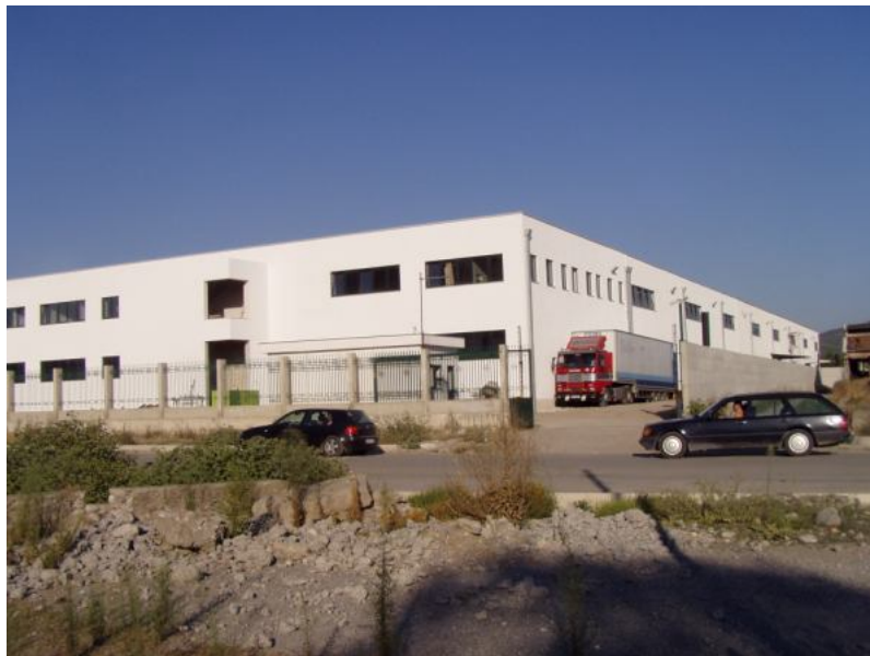
Figure 3: Building under construction in Shkodra's Industrial Zone, for a major European textile producer
